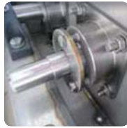
Shaft passage sealing
