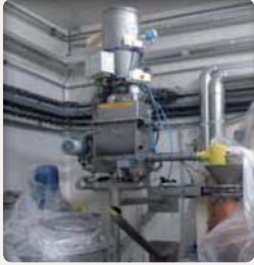
Cyclone transfer system with dosing device
