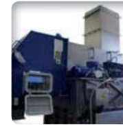
Dust collector system to vacuum fine particles.
