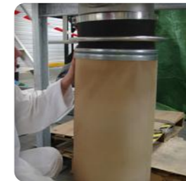
➤ Containment and sealing of filling process
