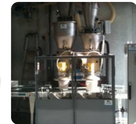
➤ Accumulation and ejection conveyors provide buffer storage and ensure the drum transfer for further strapping process.
