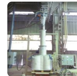
Connection to the truck loading spout
