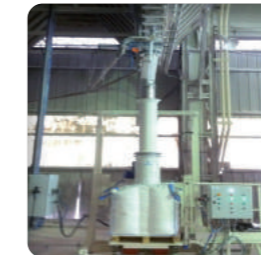
Connection to the truck loading spout
