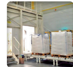
➤ Conveyor and automation
