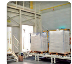
Conveyor and automation
