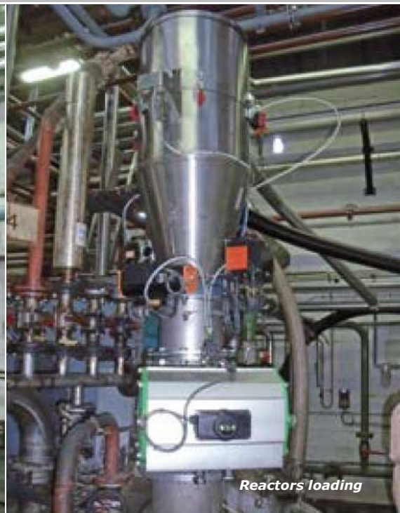
Raw materials deconditioning area
