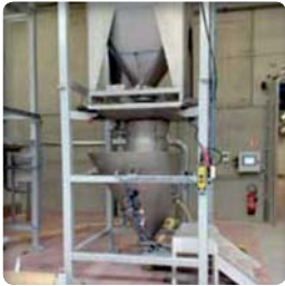
Big bag and container combined installation
