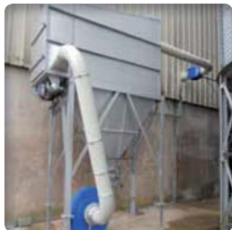
Under a dust collector
