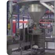
▶ Implementation on a sacks conditioning skid
