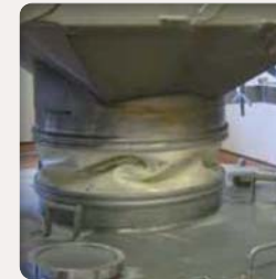
Flexible fitting on vibrating sifter
