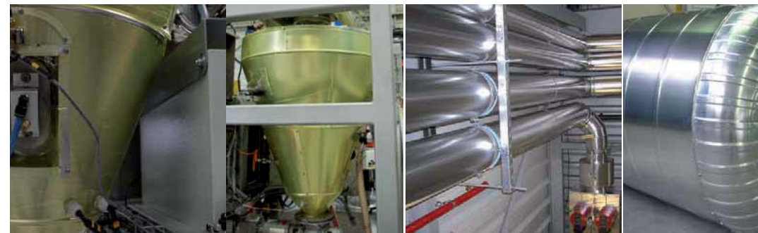
Insulated and heated hopper
