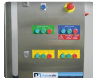
4 The control panel ensures management of doses and flow rate
