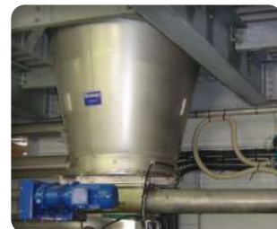
3 Feeding hopper for the storage of raw material
