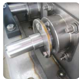
Shaft passage sealing
