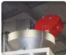
2 The explosion vent allows the evacuation of the explosion pressure
