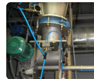
3 Dosing system for incorporation of lime
