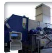
Dust collector system to vacuum fine particles.
