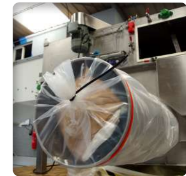
▶ Screw compactor to compact and discharge bags into a plastic sheath to secure the outlet of the compactor
