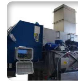
Dust collector system to vacuum fine particles.
