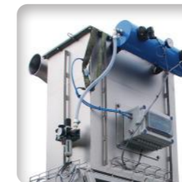
Dust collector ensuring healthy work environment
