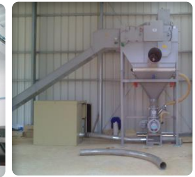
➤ Deconditioning of cement with pneumatic conveying
