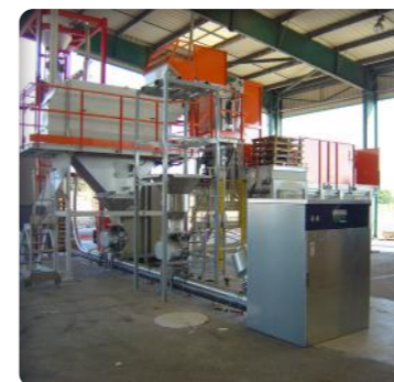
▶ Sack opening line at a polyethylene manufacturer
